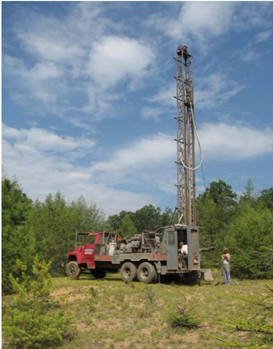
Air rotary drill rig operated by Smith Drilling in the Twomile Run watershed.
