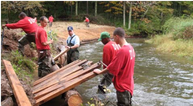
David Keller, PFBC, provides oversight to the Quehanna Boot Camp as they work on installing habitat structures.
