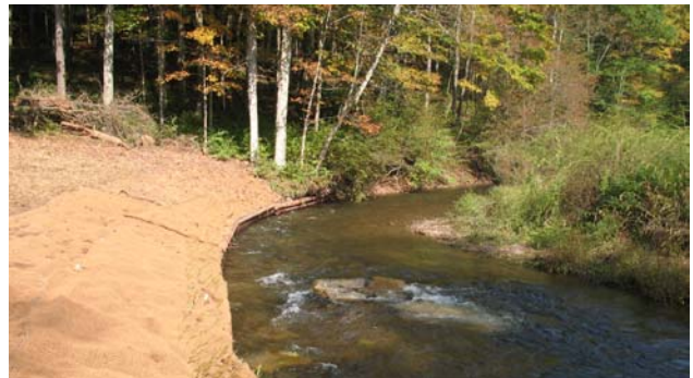
Completed mud sill and regraded and stabilized streambank shown here will provide significant habitat cover and reduce erosion.
