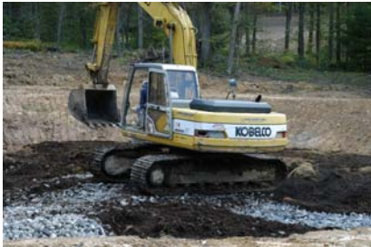
Robbins Hollow Headwaters Treatment System under construction. Photo provided by A. Wolfe
