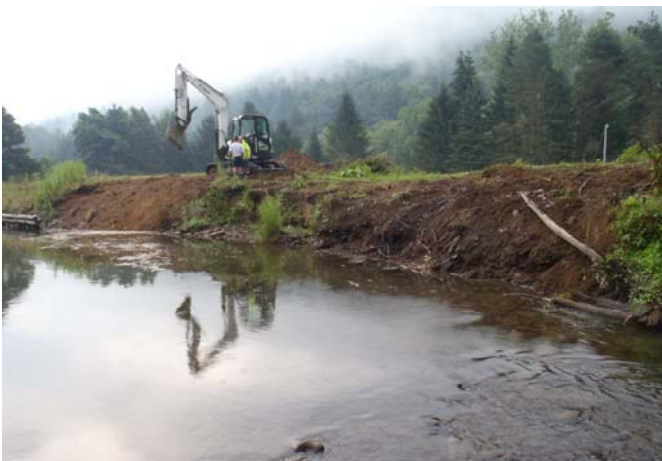
Photo shows the severe streambank erosion at the Twin Ponds project site on Kettle Creek prior to installation of a mud sill in August 2012.
