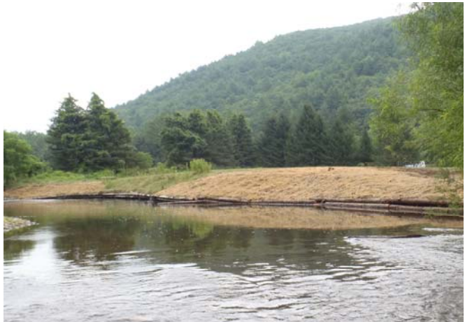
The mud sill will help to provide habitat and cover for trout during the warmer months of the year when low flow and higher water temperatures are of concerns. In combination with the regraded streambank, the mud sill will also provide additional bank stabilization.
