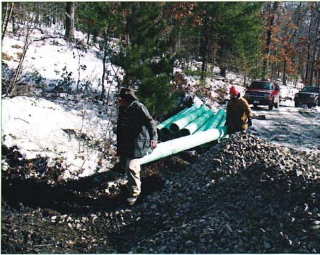
Dean Mertz (left), Kettle Creek Watershed Association Board Member, and Derek Stevenson (right) with Smith Lumber are carrying 10-inch pipe that will be used to collect the polluted water flowing from the deep mine.
