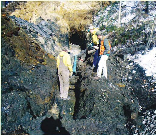
Ted Weaver (left) and Neil Wolfe (middle) of Hedin Environmental, and Bob Fitterling (right) from the DCNR Bureau of Forestry, at the collection trench where pipe is installed to directly collect the polluted flow of water from the deep mine.
