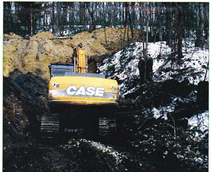
Onlookers - "Manny" Probst (left) and "Bud" Dowling (right), both of Renovo, watch the construction activities and get a peek at history.
