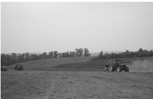
In mid-August 2004, mulch and seed were spread over the entire project site. Once the vegetation reaches 70% growth, the temporary conveyance ditches and sediment retention basins can be removed. This will likely take place in the spring or early summer.
