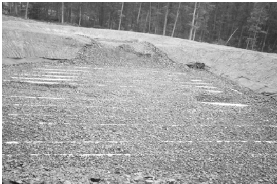
Six-inch perforated PVC pipes were installed horizontally toward the top of the limestone layer in the vertical flow ponds. These pipes are used for flushing metal precipitates from the pond.
