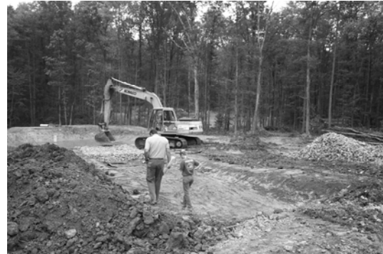
Ted Weaver (Hedin Environmental) and Amy Wolfe (KCWA/TU) inspect construction progress as E.M. Brown installs the limestone channel leading from vertical flow ponds to the settling pond (or sometimes called a flush pond).
