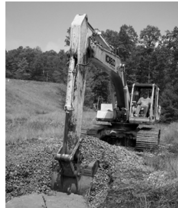
The excavator digs a pit in the limestone treatment beds in order to observe the condition of the limestone and metal precipitates that have accumulated at various depths.
