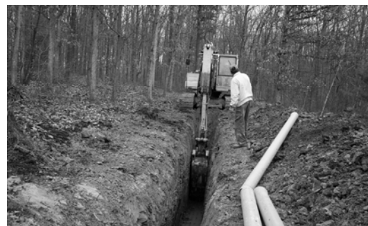
In mid-October 2004, construction began for the subsurface collection system in the "Swamp Area" downgrade of the project site. Perforated and solid pipe is installed in trenches, some as deep as 11 feet, for the purpose of collecting and monitoring the remaining flows of acid mine drainage to aid in designing a passive treatment system for the remaining discharges.
