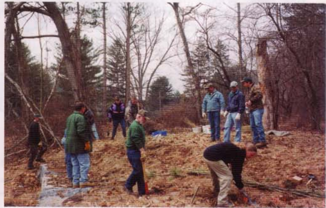
The entire fascine bundle is placed into the trench that has been dug along the contour of the regraded streambank.
