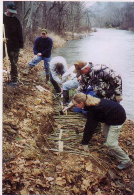
The brush layers are installed with the butt ends shoved into the bank and the tips pointing toward the stream.
