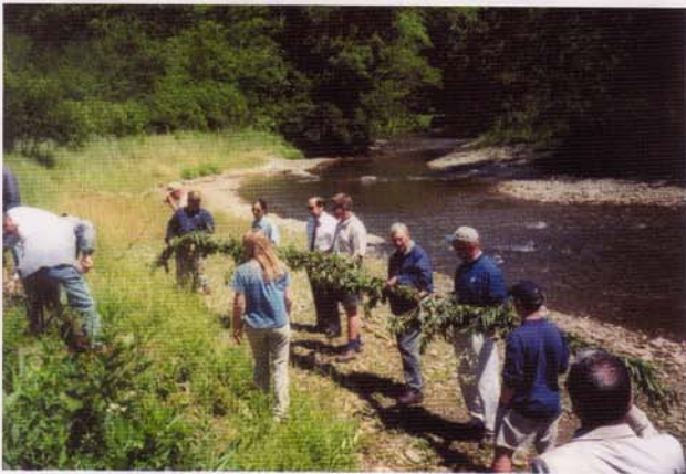
Each individual fascine bundle has been connected to another to create one long fascine bundle.
