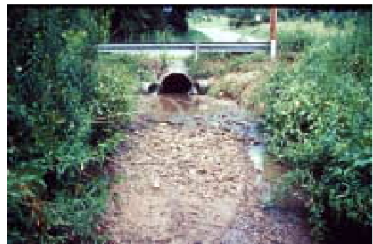
Figures 5.16, 5.17 - Road crossings can be the single largest contributor of sediment to a stream on forested watersheds. Additionally, road crossings can limit fish passage, cause localized erosion and be a costly maintenance problem after floods. Stream crossings are listed by subwatershed in the chart above for comparison.
