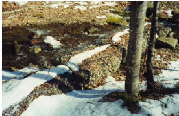
Gabions along Elk Lick Run
