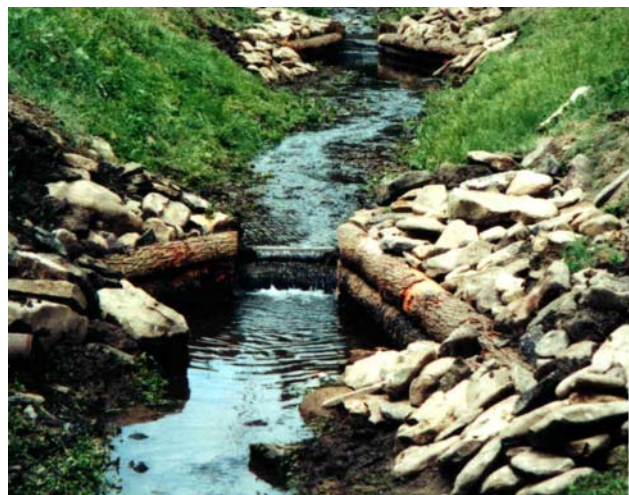
Close-up view looking at the downstream wings installed below one water jack dam on Germania Branch.
