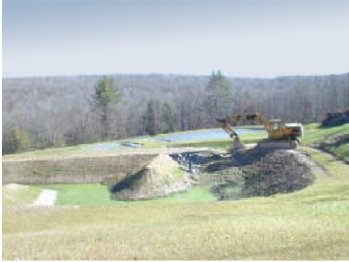
Passive AMD treatment system near completion on Middle Branch in the Twomile Run subwatershed. Passive systems, like this vertical flow pond will be, implemented in other parts of the Twomile watershed.
