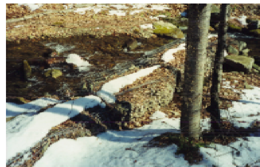
Gabion on Elk Lick Run
